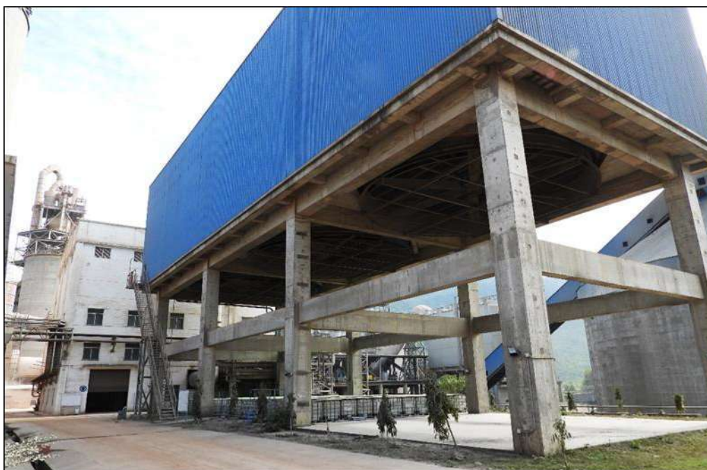
Figure – 3: WHR System in STC Cement Plant
